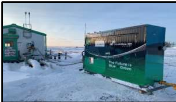
TOU diesel displacement with NG
