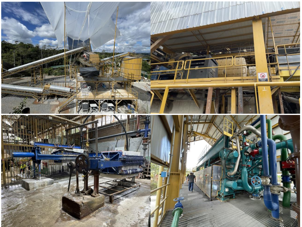
Figure 7: (clockwise from top left) New crushing facility, Ball mill, New filter press in tailings treatment facility, Merrill Crowe system, Filter presses in front of the smelting room
